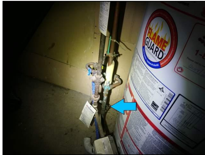
Main water shutoff valve
