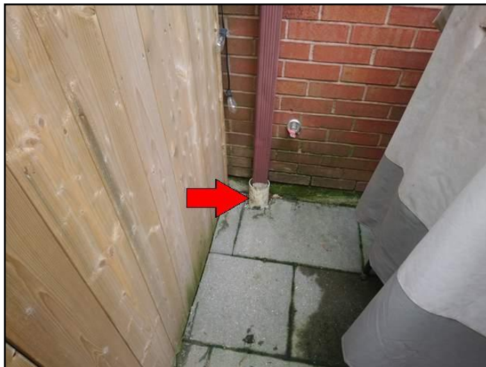
Ex: Below-grade discharge noted
