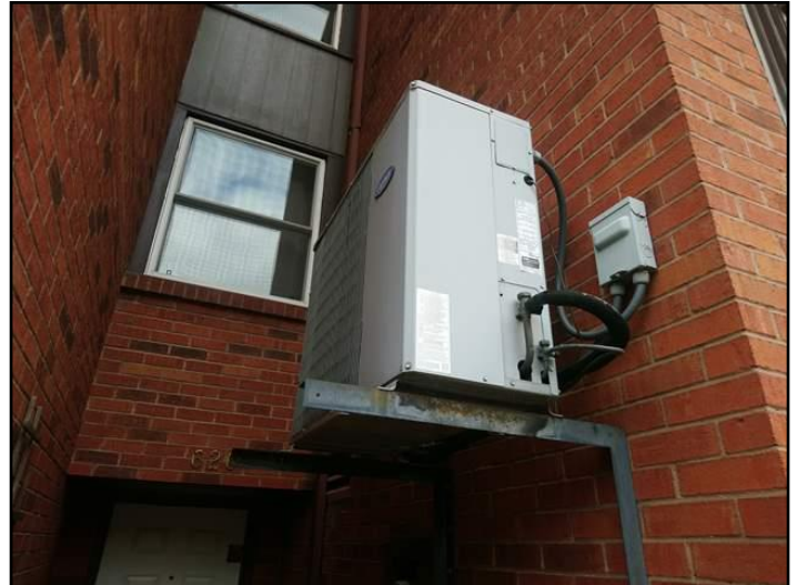
Air cooled condenser
