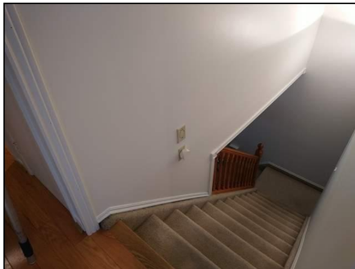
Handrail incomplete / not continuous
