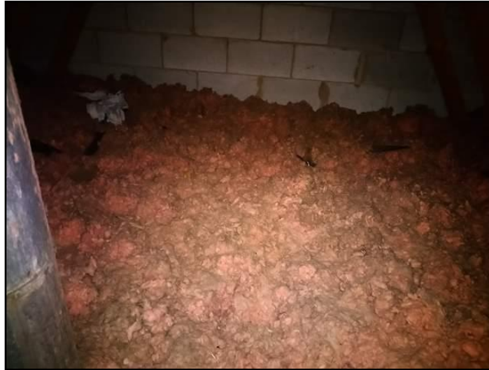
Fiberglass attic insulation
